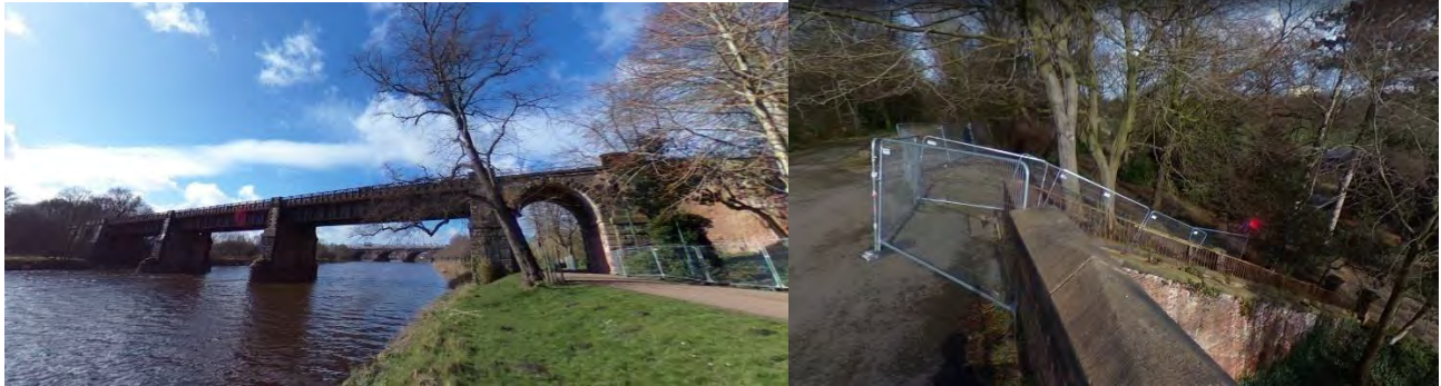
Figure 2-16: Avenham Viaduct bridge, left, with damaged staircase and footpath posing risk to the structure, right
